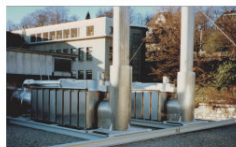
1988: First urea operated DeNOx plant, 4.4 MW, EW Schaffhausen
